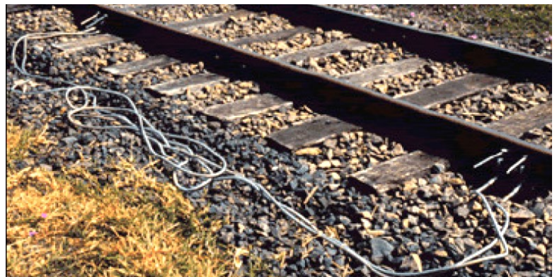
Figure 2: Example of duplicate temporary traction bonds installed before cutting traction rails in electrified corridors.
