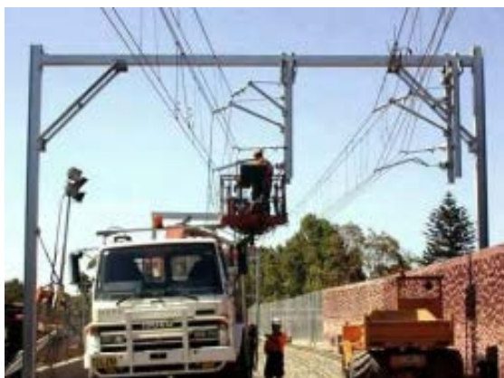
A signal portal
